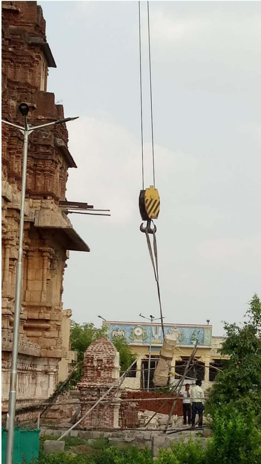
A mammoth 300 tonne crane capable of lifting 30 tons to 150 feet height was in operation handling the massive Granite pillar.
