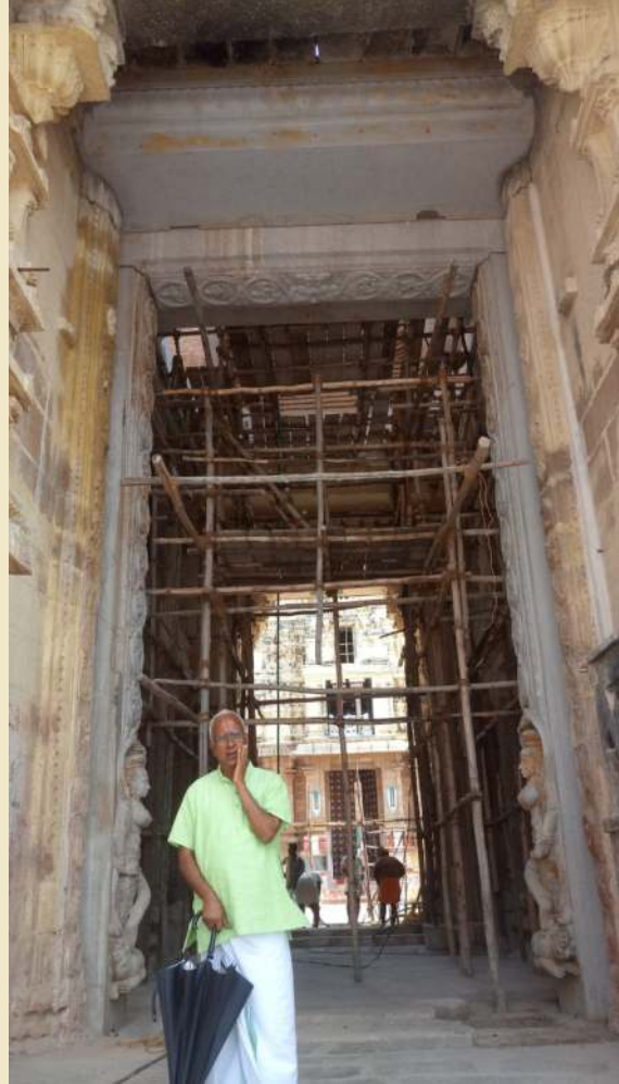
After five years of extensive renovations from 2014 to March 2019, the main RajaGopuram entrance, 10 feet width x 20 feet height was restored to its original Grandeur
