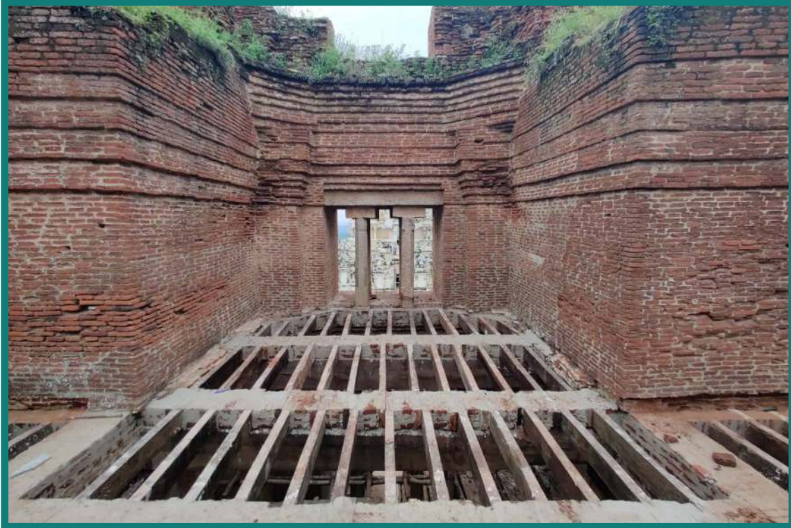
The 1st Tier (முதல் நிலை) Madras-Terrace, Granite stone pillars, Illuppai wood beams and rafters are placed in position, capable of receiving the Lime-Mortar and the special brick structure.
